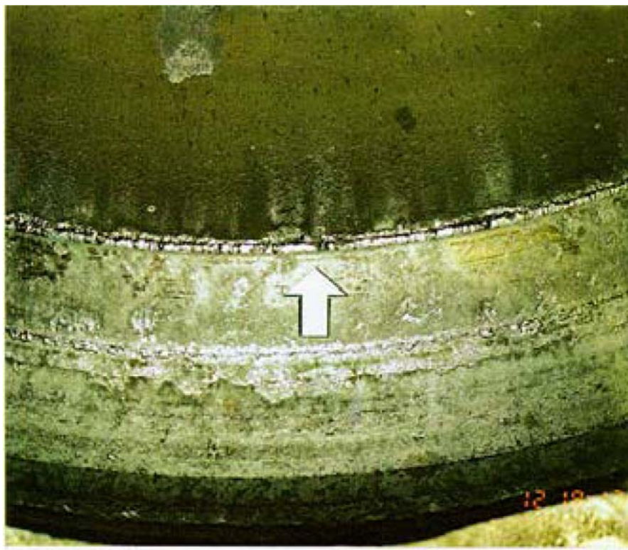
Photo 2: Minor leakages, and “fans”
